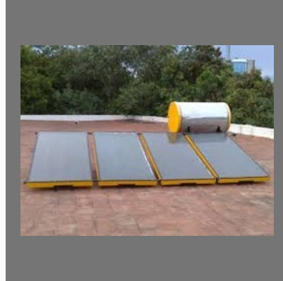
Industrial Solar Water Heater
