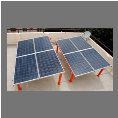
Solar Rooftop System
